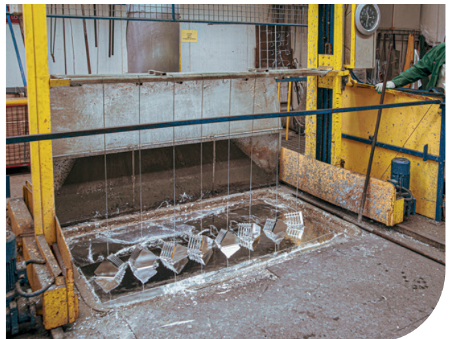
Hot-dip galvanizing plant (2003)
